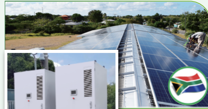
TAICO 430KWh Storage Installation in South Africa System Capacity:2 x215KWh Model: TK E-Cube L200
