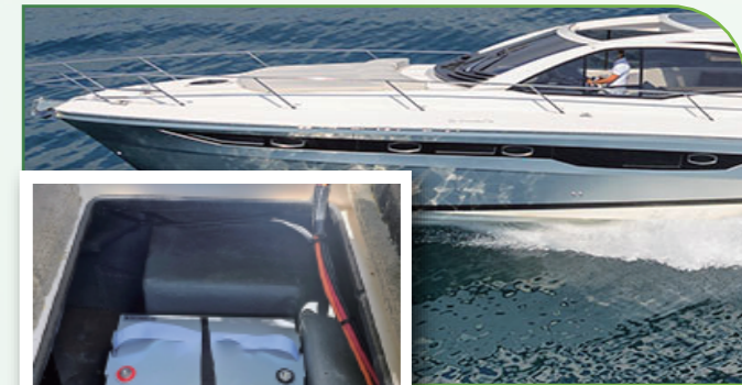
Yacht battery install Model: LFP12V-100
