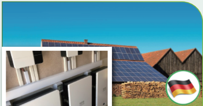
TAICO 51KWH Storage Installation in Germany System Capacity:10 x5.12KWH Model: TKPW 2400
