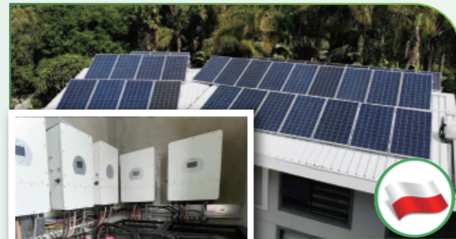
TAICO 92KWH Storage Installation in Poland System Capacity:6x15.36KWH Model:TK1500
